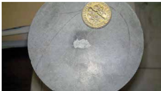
Fig. 2: Close-up of typical flaked area on slab placed in 2012. Note that the nearby surface is darkened and exhibits craze cracking. For scale, a U.S. dime is about 0.71 in. (18 mm) in diameter
