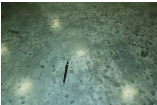
Fig. 4: Surface distress may occur over a wide contiguous area (in this case, the distress covered about 400 ft 2 (37 m 2 )). This surface is shown after about 1 year of service, prior to repair
