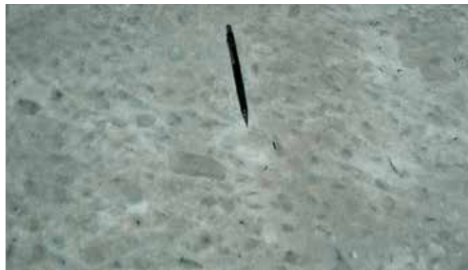
Fig. 1: An example of aggregate shading on the surface of a 10 in. (250 mm) thick floor constructed in 2007. The mixture used on this project comprised large aggregate with very elongated top-size particles, nominally 4 x 1 in. (100 x 25 mm). While the unusual aggregate made it a challenge to achieve adequate embedment, flaking of the surface was observed only in a very limited area
