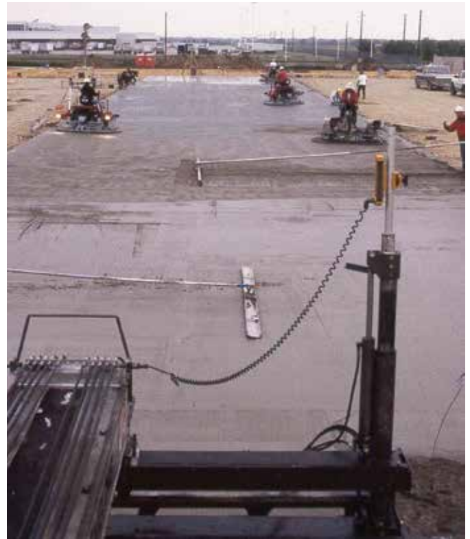
Fig. 7: Typical industrial slab finishing steps: laser screed (fore-ground), bull (channel) floating, check rod, power floating, and power troweling (photo courtesy of Structural Services, Inc.)
